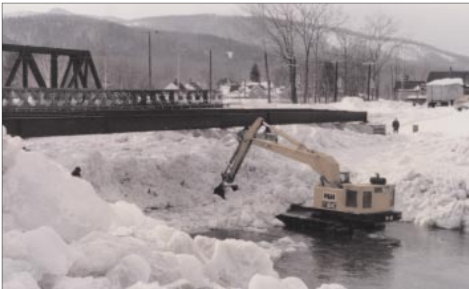
Figure 7. Backhoe clearing channel in Peabody River, Gorham, New Hampshire, February 1982. (Photograph by Dan Ayer.)
