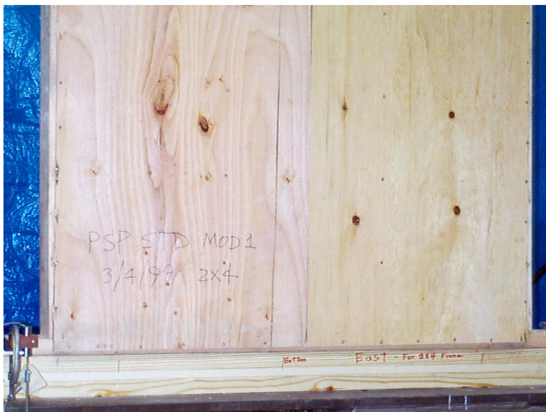
Figure 84. Bottom of the PSP-Std-MS1 panel showing plywood to stud nail connection failure.
