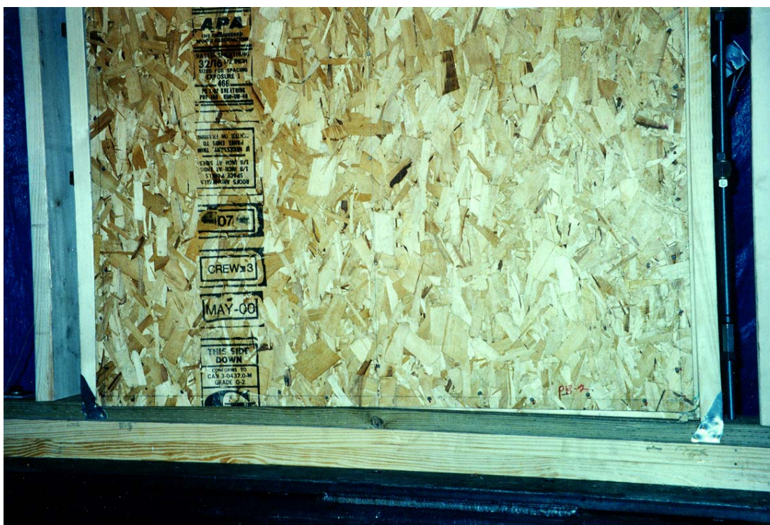
Figure 38. Gap in inset panel due to nails yielding in OSB to panel connection.
