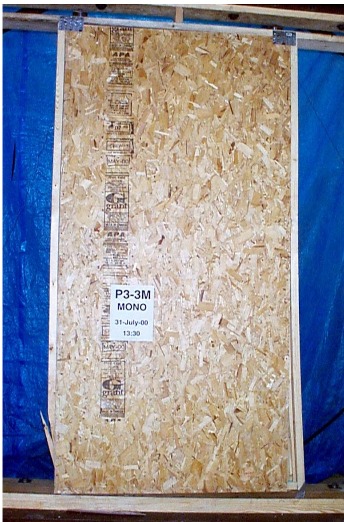
Figure 54. Overall view of damaged P3-3M mono test panel.
