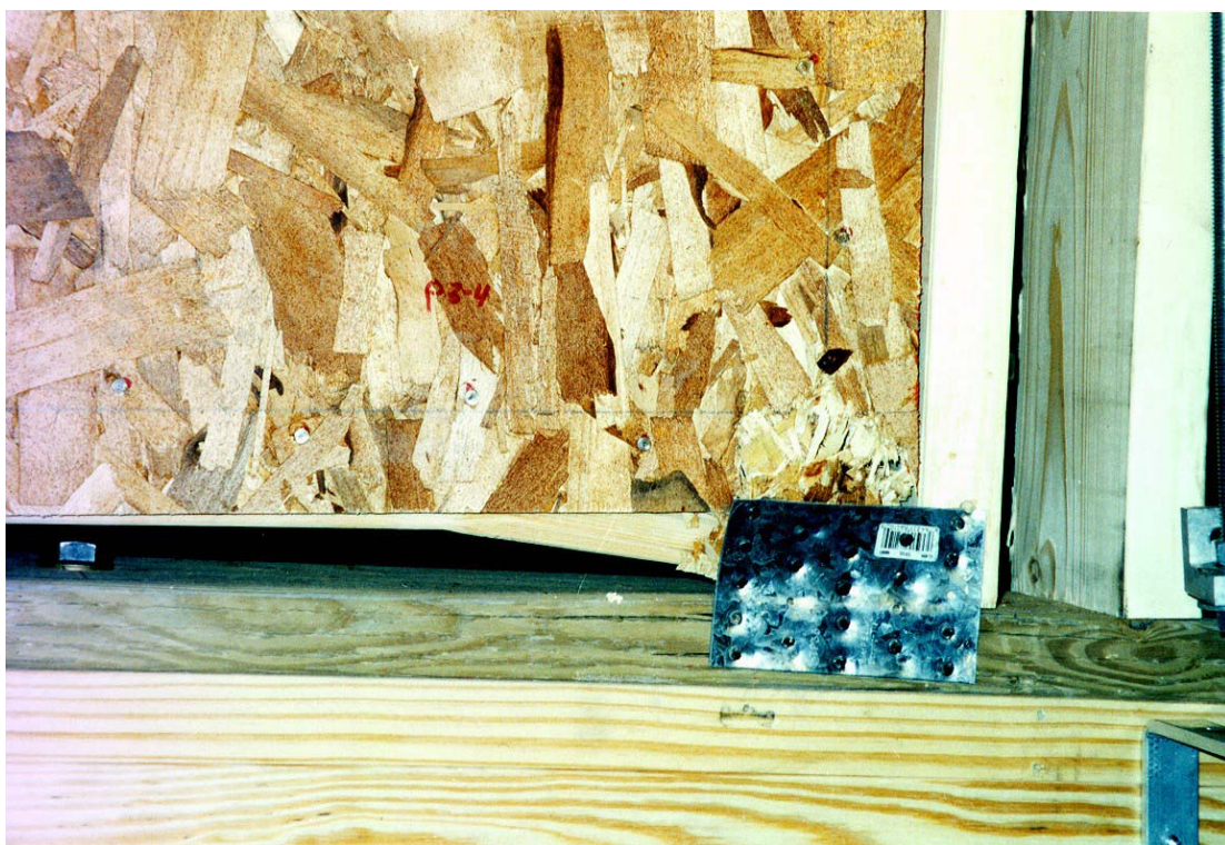
Figure 47. Damage to OSB and inset panel bottom plate at right corner of P3-4 mono panel.
