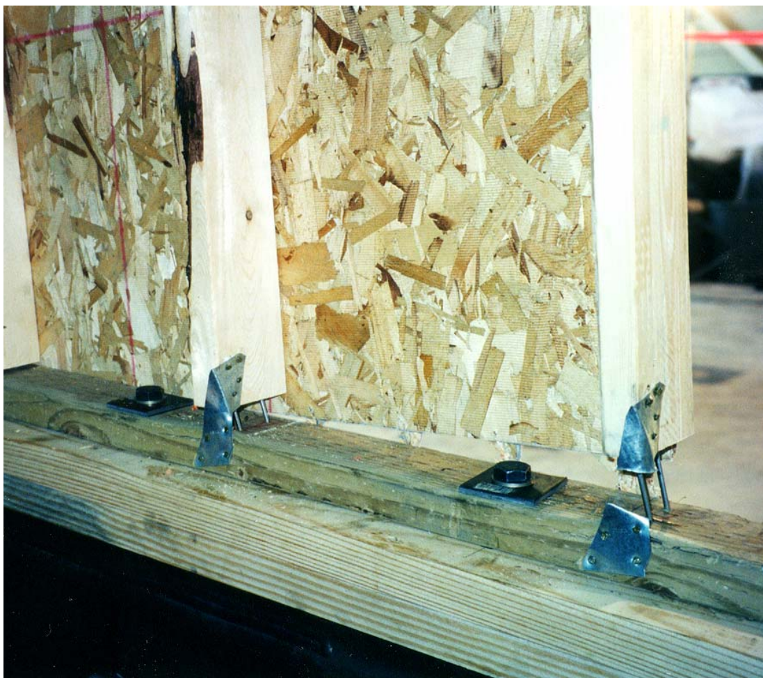
Figure 70. Shear failure of hurricane tie and nail yielding.
