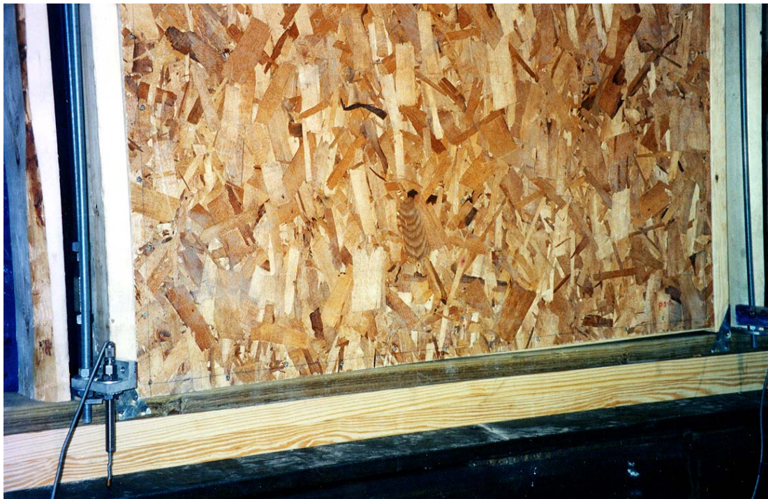
Figure 33. Gap at bottom of panel (right side) due to nail yielding.
