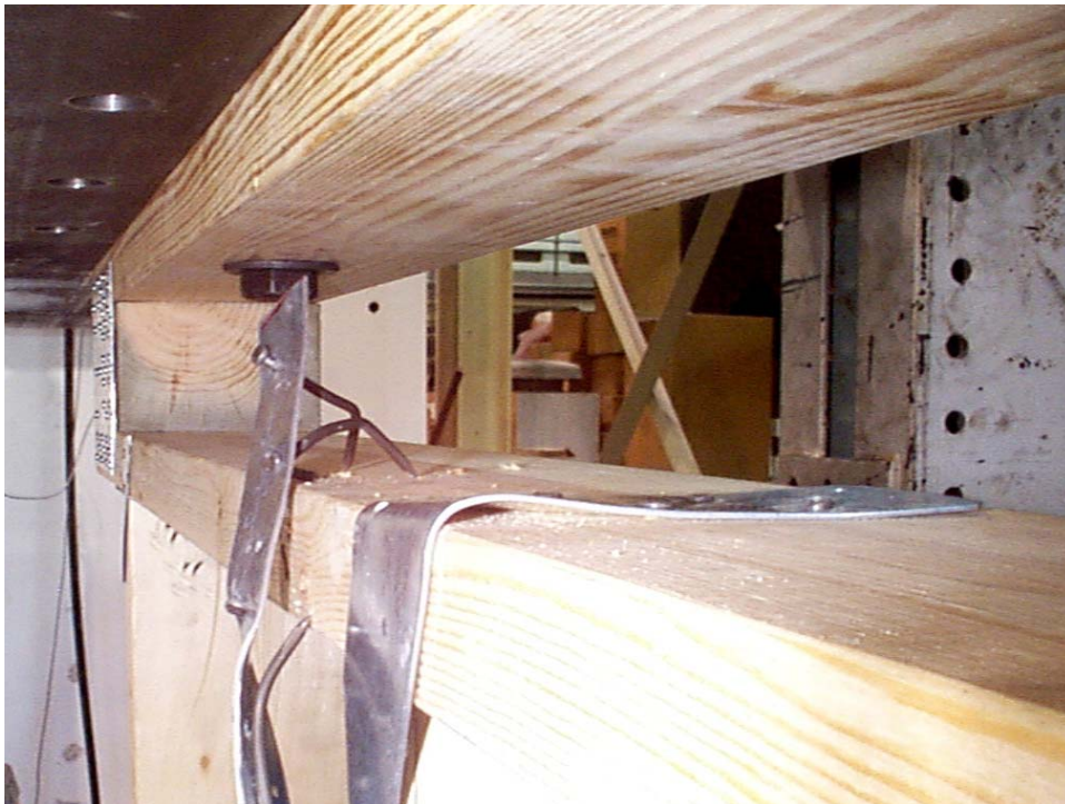
Figure 25. Nails attaching steel strap to top plate yielded and pulled out.
