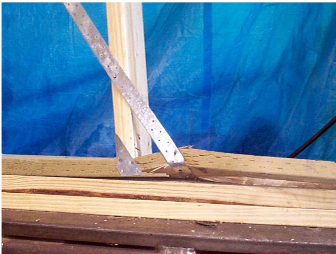
Figure 29. Damage in bottom plate due to tensioning of steel strap.
