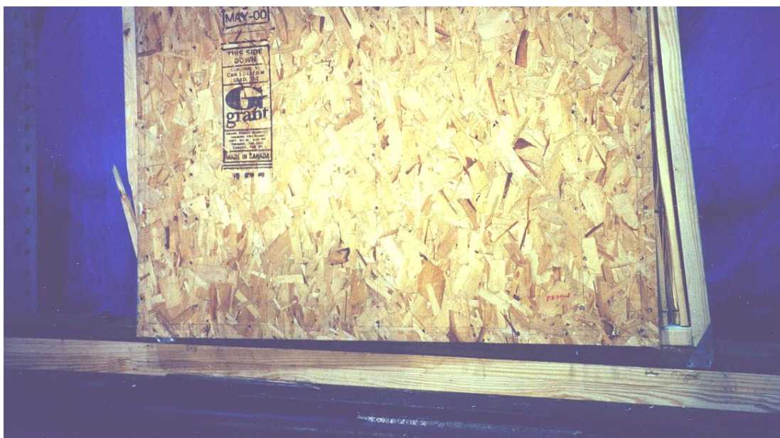
Figure 55. Bottom of P3-3M mono panel showing the OSB pulled away from frame.
