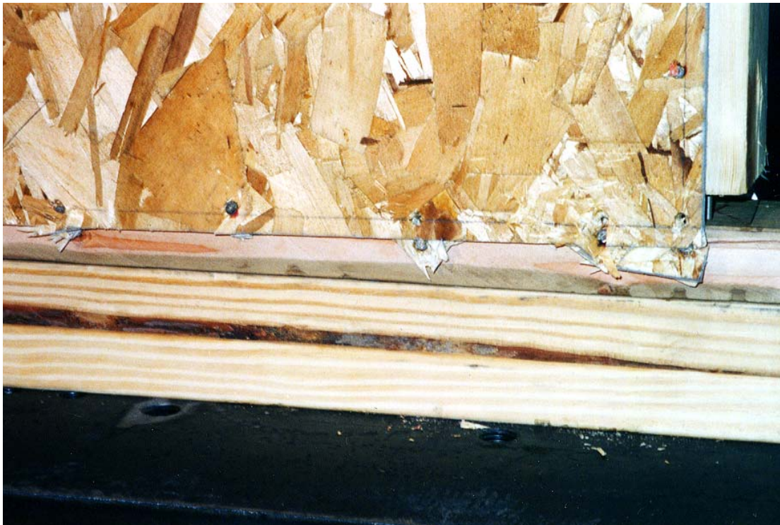
Figure 72. Nails pulled through bottom right corner of the OSB of P3-6 CUREE1 panel.
