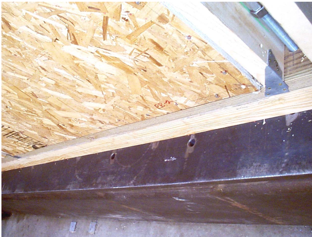
Figure 39. OSB pulling out of frame in lower right corner.
