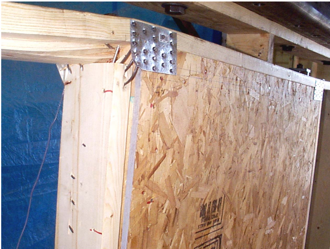
Figure 52. Splitting and bending failure of P3-5 mono top plate.
