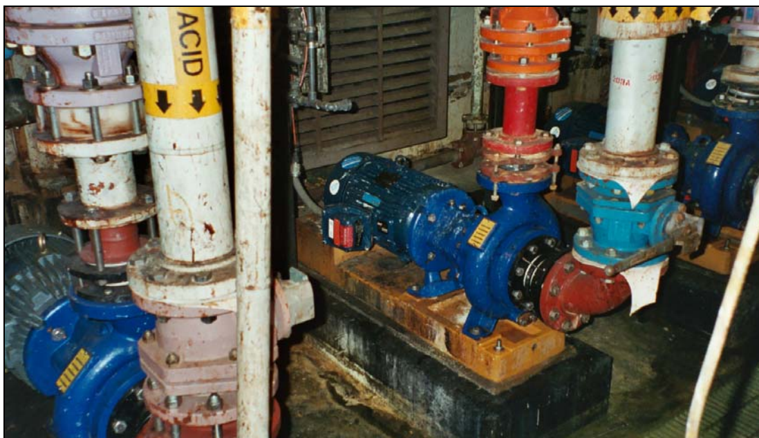
Figure 19. New magnetic drive sealless chromic acid pumps.
