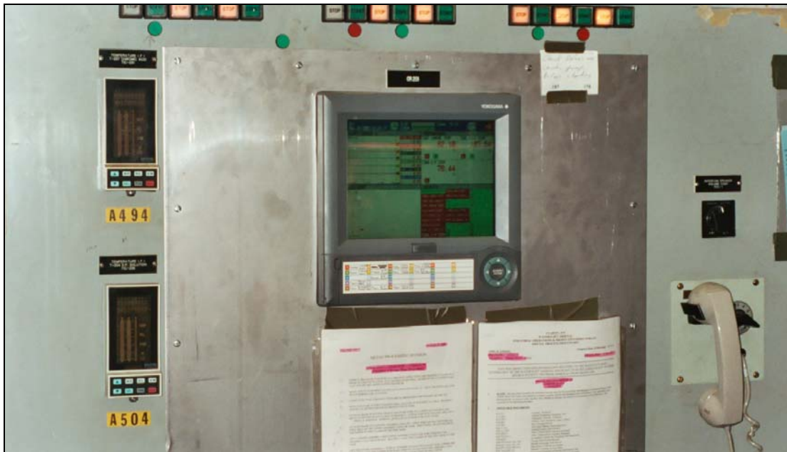
Figure 12. DX200 in service, control panel CP-201, 120-mm plating area, Bldg. 35, WVA.
