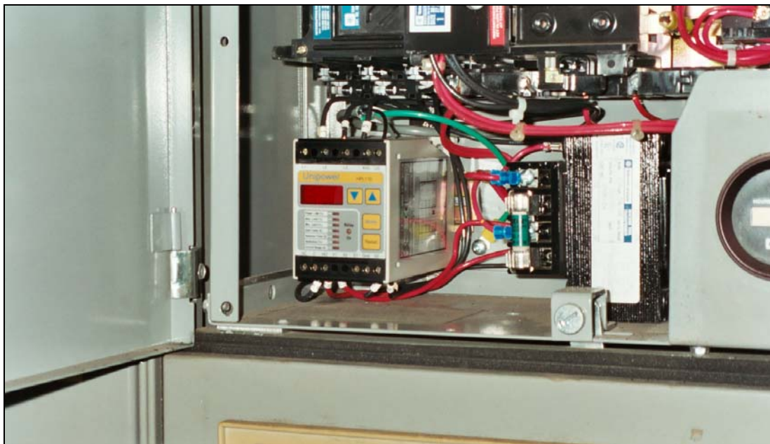
Figure 22. Power monitor, MCC starter bucket for electropolish pump.
