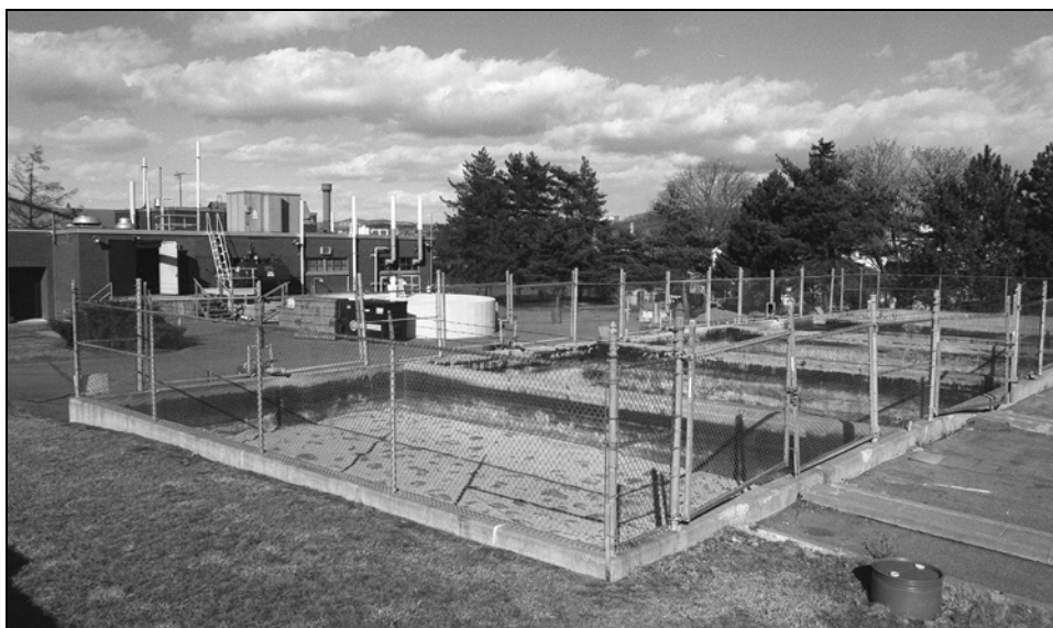
Figure 10. Industrial Wastewater Treatment Plant at WVA.
