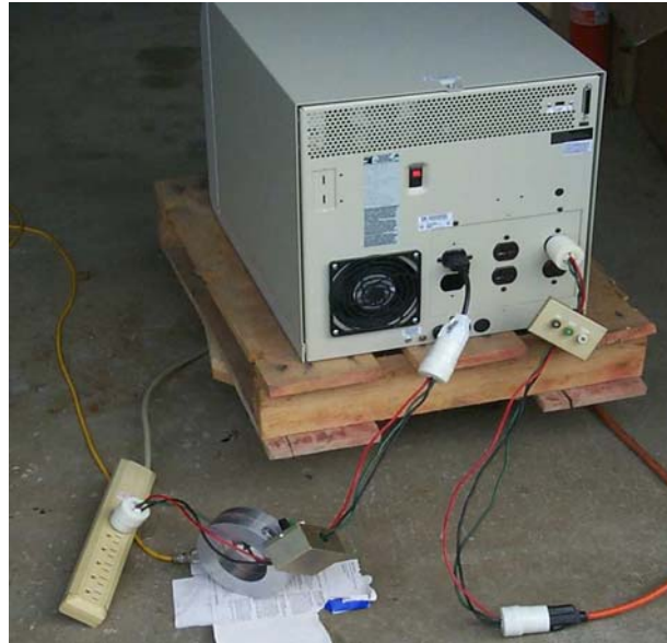
Figure 3.5: UPS under Test
