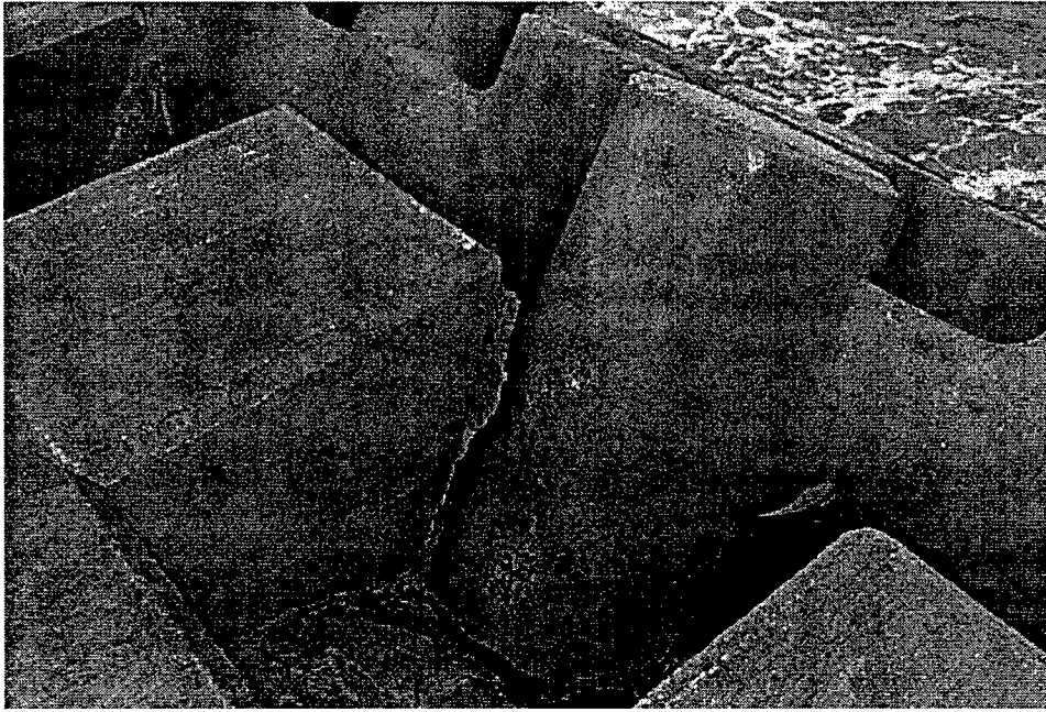
Figure 11. Separation between tribar and rib cap
