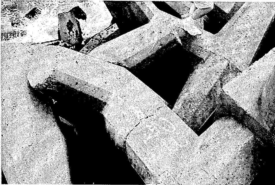
Figure 28. Dolos with mid-shank crack
