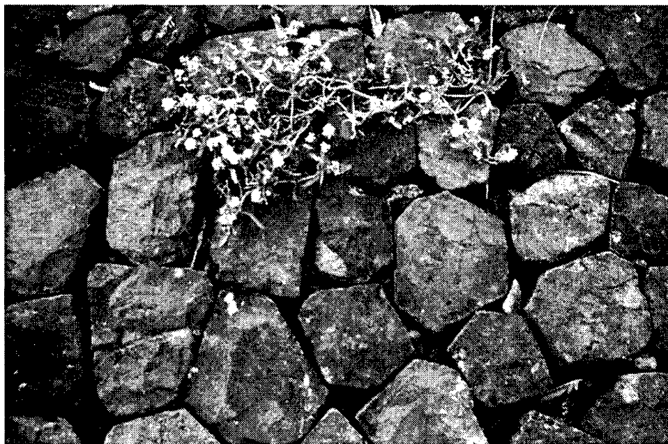
Fig 13. Vegetation growing through a rock revetment
