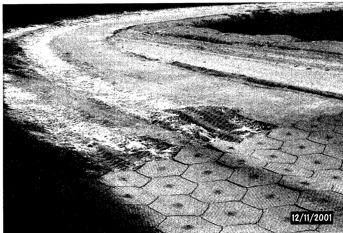
Photo 82. Deterioration in the transition zone
