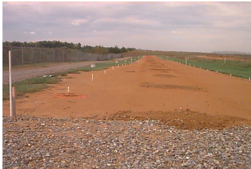
Figure 17. Site 12 mine, sand.
