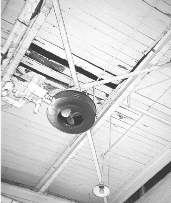
Figure 8: Ceiling fan in bathroom (ERDC/CERL).
