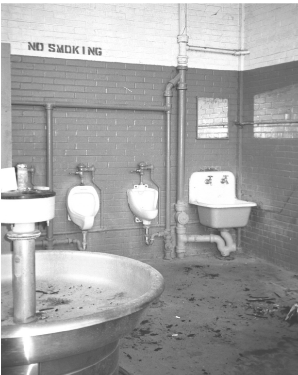
Figure 9: Bathroom fixtures, including the Bradley Wash Fountain (ERDC/CERL).
