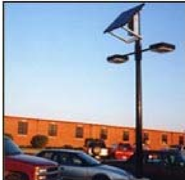
Figure 18. Solar parking lot light.
