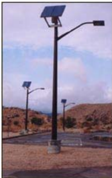
Figure 17. Solar parking lot lights.
