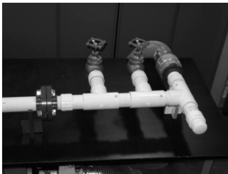
Figure 19. Exit duct bypass valves
