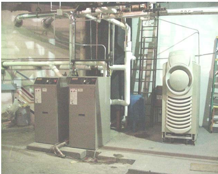
Figure 7. Fort Drum microturbine and DHW heaters.
