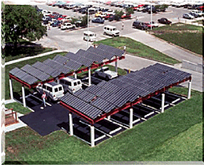
Figure 10. Photovoltaic Panels over Parking Lots
