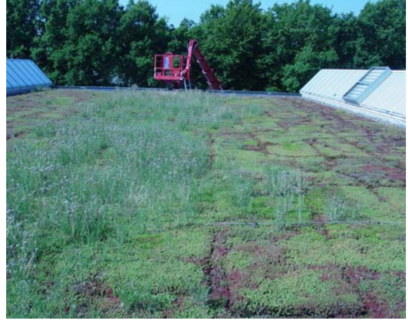
Figure 4.10 Oldenburg Bus Station. Wild onions have grown in the low spots near the drains
