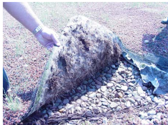
Figure 4.20 Building 3. Only sedums remain on the portions of the roof with only gravel and no soil.
