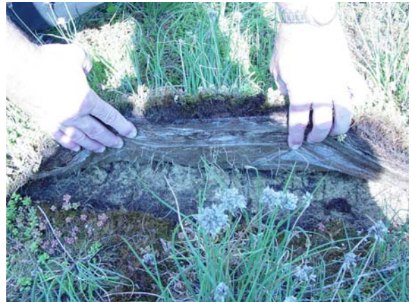
Figure 4.12 Green Roof Mats. No growing medium was used on this roof except the substrate in which the mats were grown before installation.
