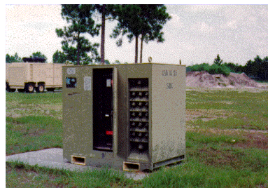
Figure 14. Secondary Distribution Center
