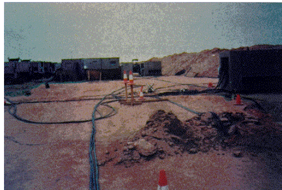
Figure 19. Typical Above Ground Electrical Distribution.
