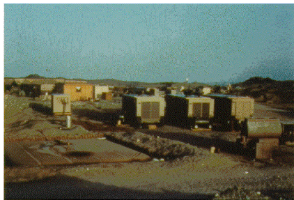
Figure 15. Power Plant Set Up.
