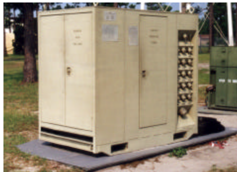
Figure 9. Secondary Distribution Center.
