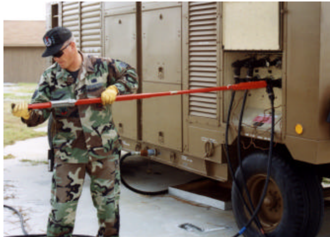
Figure 59. Use of Grip-All Clamp Stick for Connecting to Generator.
