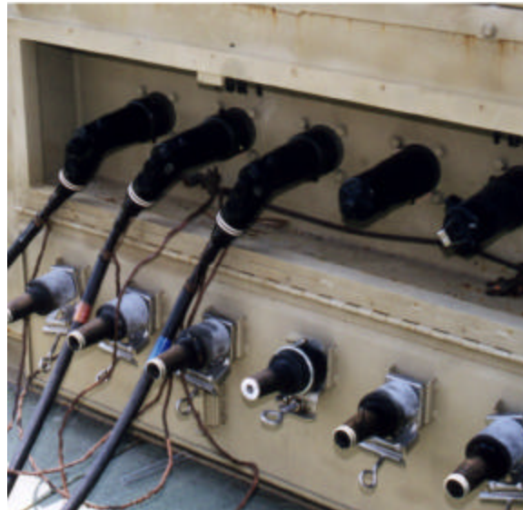
Figure 49. PDC Output Ground Connection.
