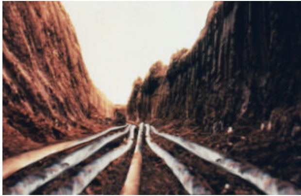
Figure 47. Multiple Cable Runs in Common Trench.
