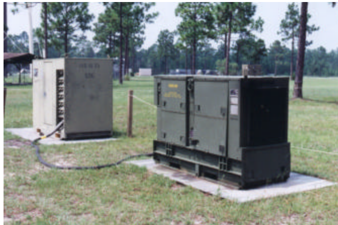
Figure 10. SDC with MEP Cable.
