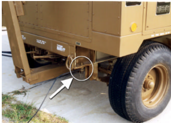
Figure 39. Ground Stud on MEP-12A Generator.
