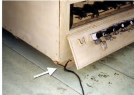
Figure 40. Grounding Locations on the PDC.
