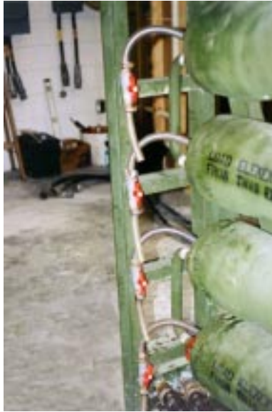
Figure 35. Front R.O. Pressure Tube Vent/Sample Valves.
