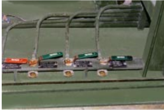
Figure 42. Cartridge Filter Drains #1 and #2.
