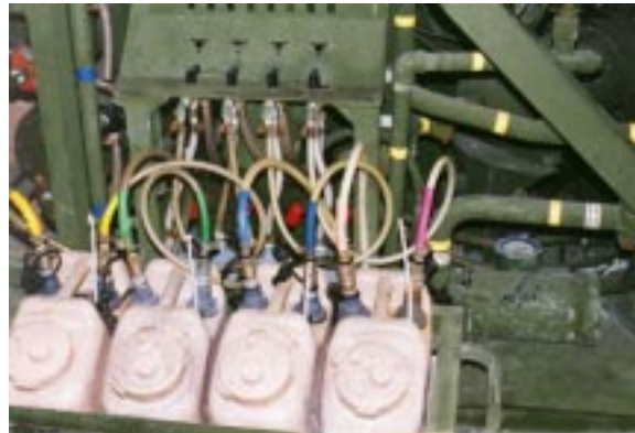
Figure 30. Chemical Feed Can Connections.
