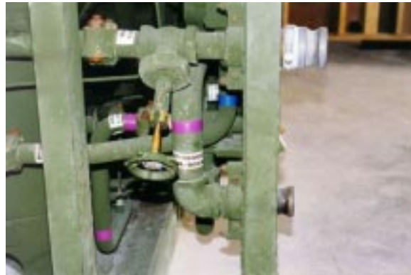
Figure 33. VENT VESSELS Gate Valve.
