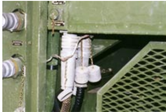
Figure 31. Electrical Power Connections at Junction Box.
