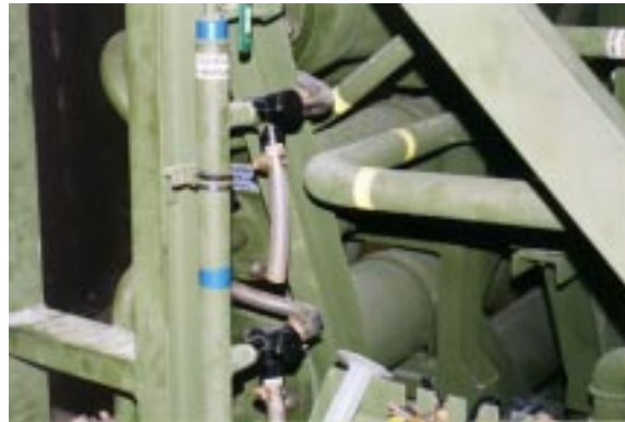
Figure 36. Rear R.O. Pressure Tube Vent/Sample Valves.
