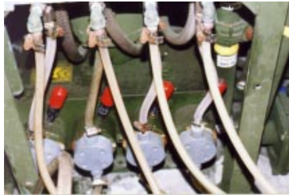
Figure 9. Chemical Feed Pump.
