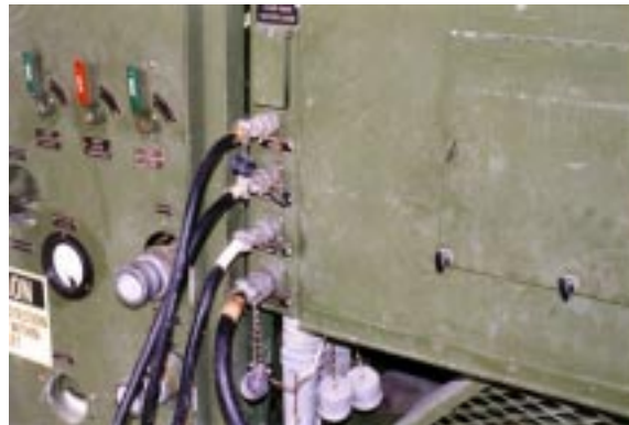
Figure 26. Electrical Connections from Raw Water Pumps to ROWPU.
