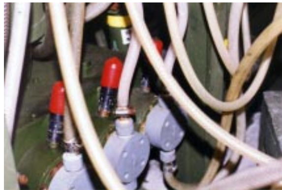
Figure 38. Chemical Feed Pump Controls.
