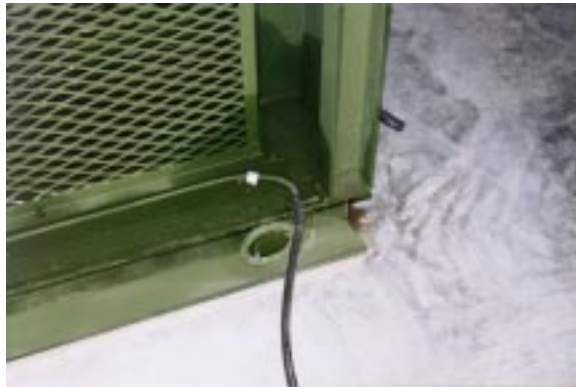
Figure 39. Vent Pipe for the Three Vent Valves.
