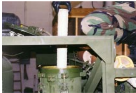
Figure 44. Cartridge Filter Tube Replacement.
