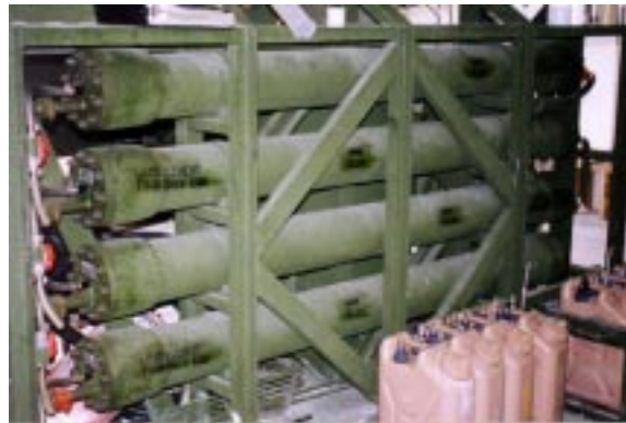
Figure 2. Reverse Osmosis Pressure Tubes.
