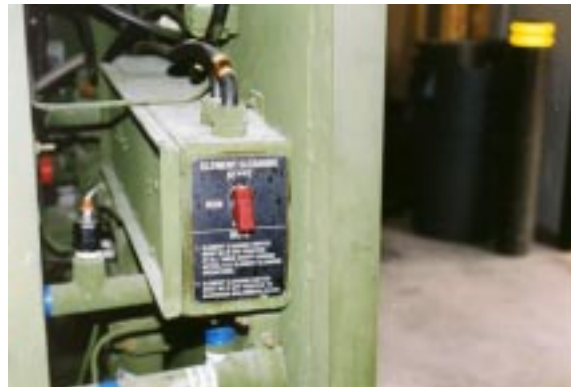
Figure 41. R.O. Element Cleaning Switch.
