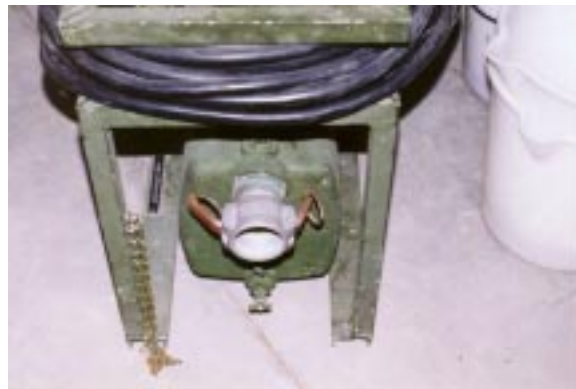
Figure 22. Fittings Attached to Raw Water Pump #1.
