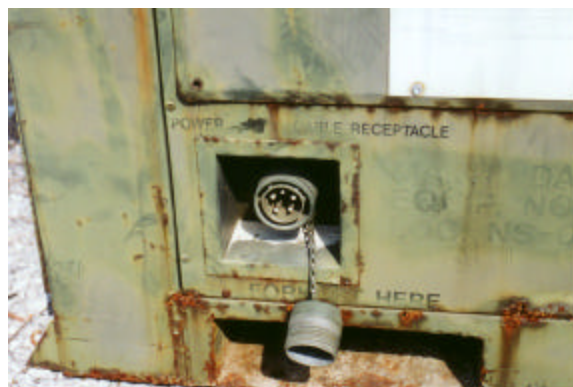
Figure 32. Electrical Connection Receptacle.
