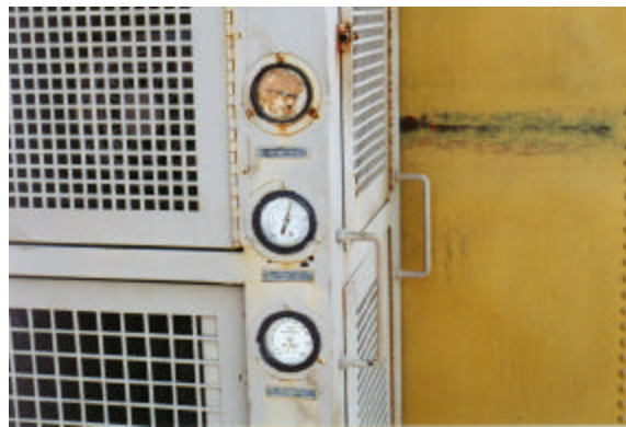
Figure 38. Temperature and Pressure Gauges.
