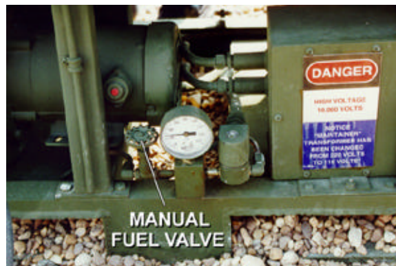
Figure 16. Manual Fuel Valve.
