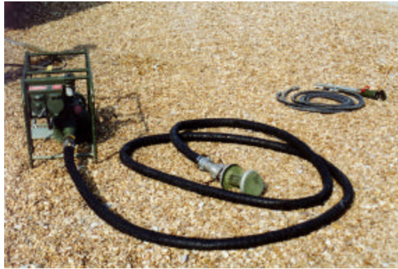
Figure 3. Water Pump and Suction Line.
