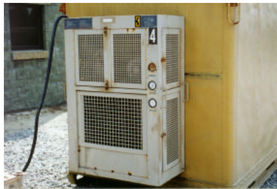
Figure 36. Mechanical Refrigeration Equipment.
