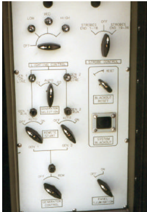
Figure 25. Primary Control Panel (Trailer #1).
