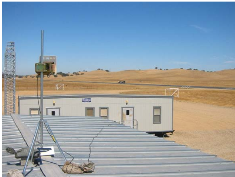
Figure 22. Base Station Sector Antenna Overlooking Runway
