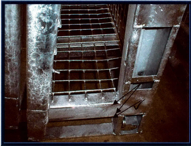
Photo 29. Bent Wire Mesh on the Interconnected ISTF-2 Units.
