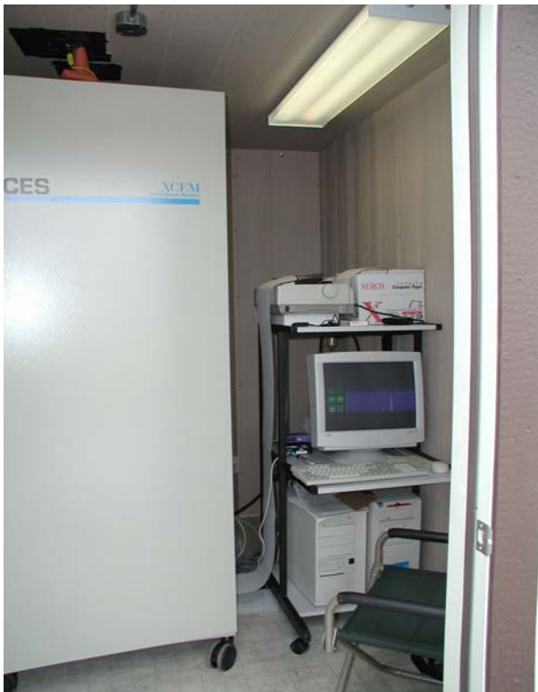
Figure 33. XCEM with computer system installed at TEAD.
