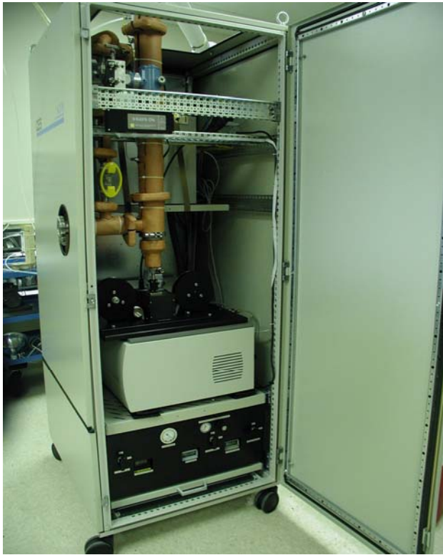
Figure 32. XCEM with cabinet door open.
