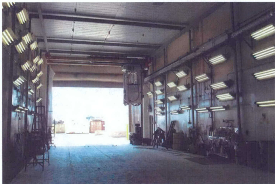
Figure 2-1. Paint Spray Booth at Ft. Hood Army Base, Texas.
