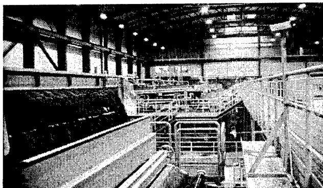
Figure 4. Parallel press installation and cake discharge
