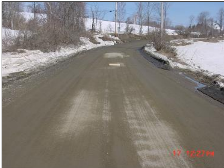
Figure 40. Cement section on March 17, 2003, showing drying compared to the CE (in the background).
