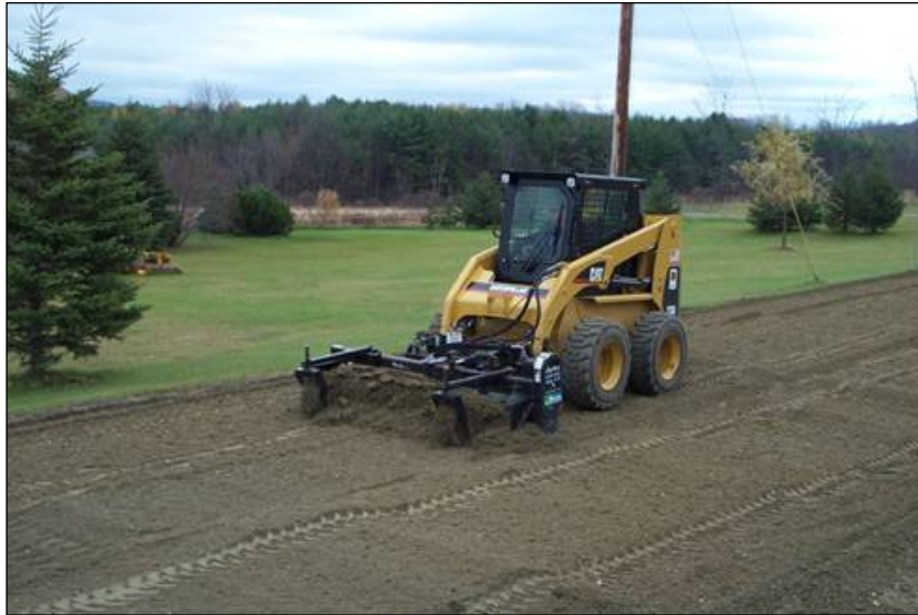
Figure 20. Westford Cement test section during construction, showing original road surface material being mixed with cement to a depth of 8 in.
