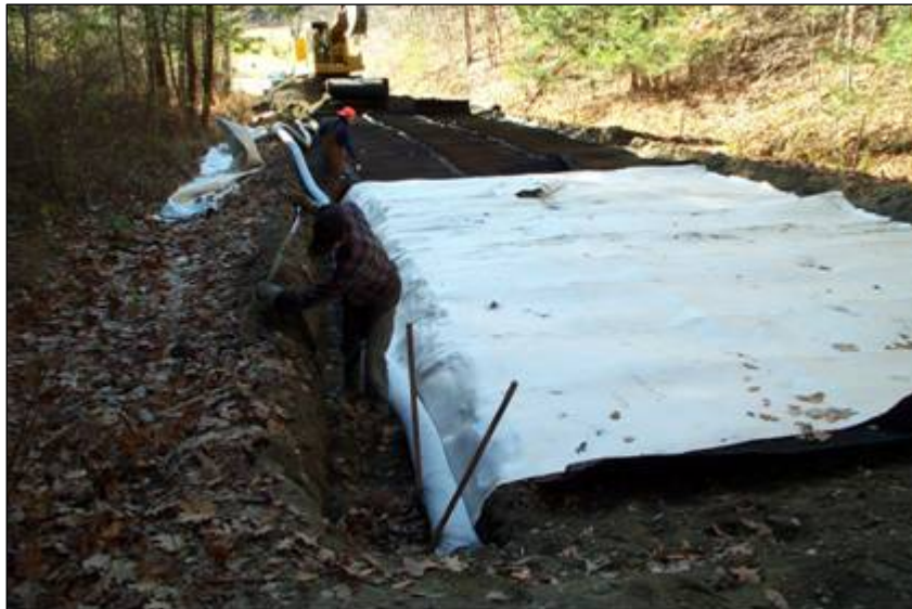
Figure 14. G CBD during construction in Windsor, Area 4. Here the transport layer (white fabric) is being connected to drain pipe.
