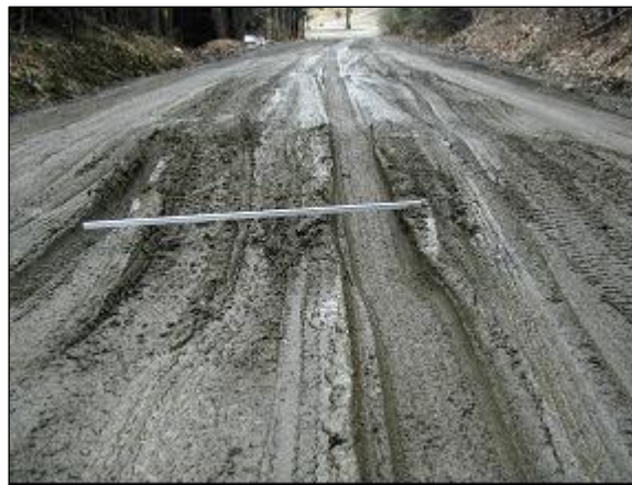
Figure 30. Area 4, looking west, after about 6 in. of “gravel” was added on April 2, 2002. Adding the gravel resulted in deeper ruts.
