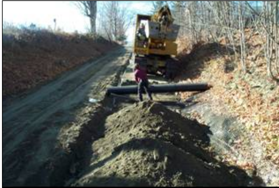
Figure 10. Installation of geogrid in Windsor, Area 2. The image is looking west; the eastbound lane was constructed first.
