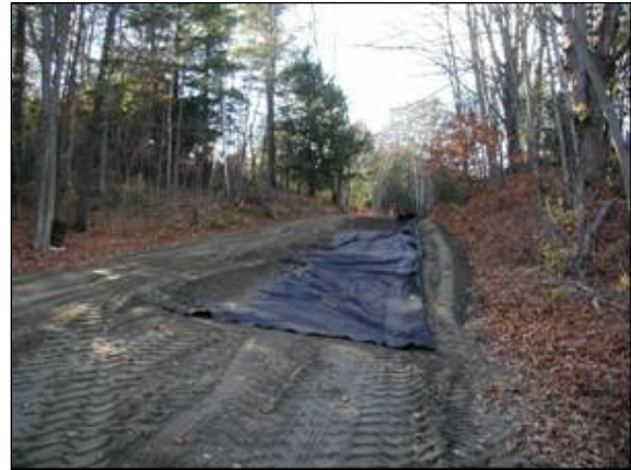
Figure 9. Geotextile separator in Windsor, Area 1, during construction. Note that there are numerous wrinkles.
