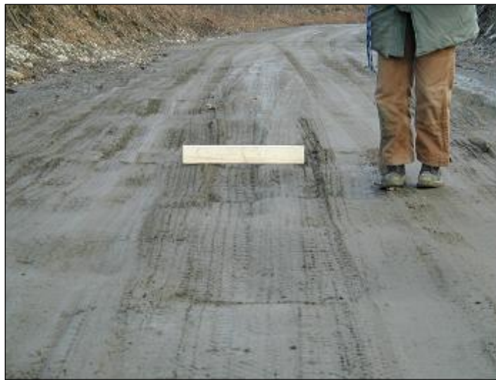
Figure 35. Corrugations and potholes on the Grid section, Area 2, March 4, 2002. The Drain section is visible in the background, showing little surface distress.
