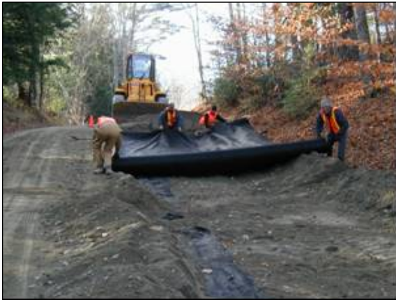
Figure 8. Installation of geotextile separator in Windsor, Area 1. Note “windrows” at edges where surface material was removed.
