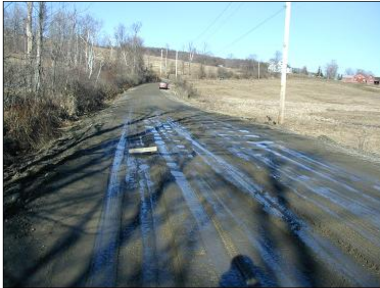
Figure 39. CW (foreground) and Geowrap sections (background) on March 11, 2002. The CW ends and Geowrap section begins at the location where the soil transitions from wet to dry.
