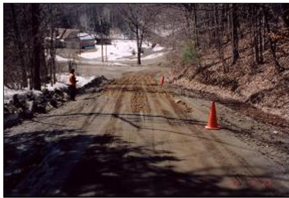
Figure 41. CW of Area 4 on March 24, 2003, showing its sunny exposure. The orange cones mark the ends of the test section. Note that new material was added to this section. The GCBD section is in the foreground.
