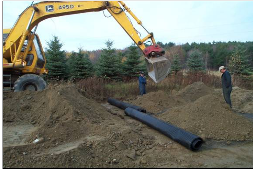
Figure 19. Westford Geogrid test section during construction, showing original road surface material being placed on the grid.
