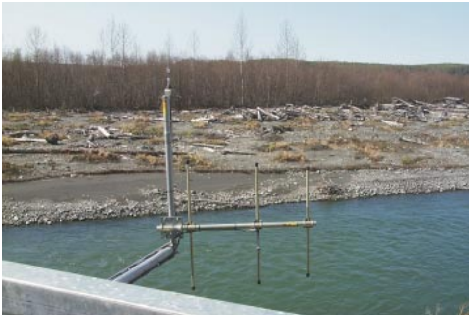
Figure III-5-6. Base station antennas.
