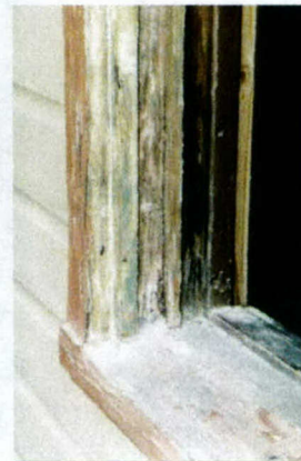
b. stripped corner
