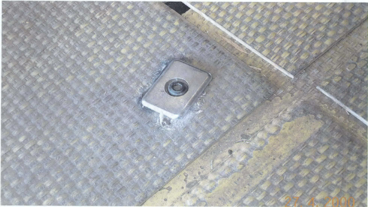
Photo 38. Movement of MP Mat pin within connection. Pin did not fail. (Low-strength soil, 3 to 5 CBR)
