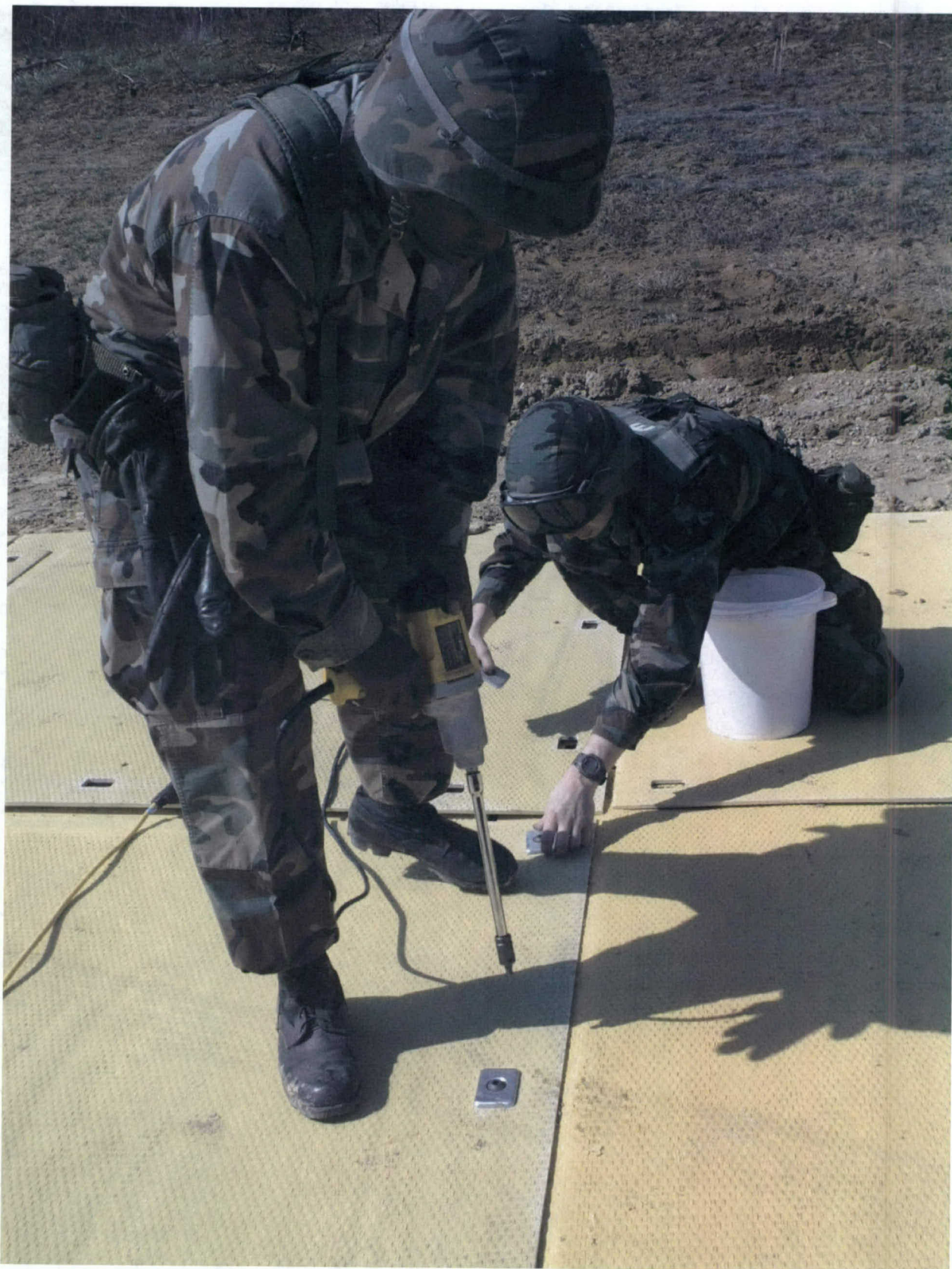
Photo 17. Placing MP Mat connector pins and locking pins with electric impact wrench
