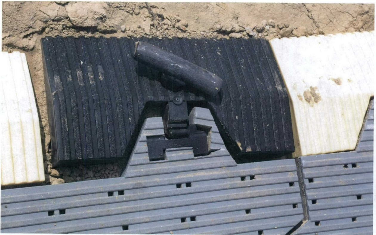
Photo 24. Isolated structural damage to SUPA-TRAC matting system at helipad edge
