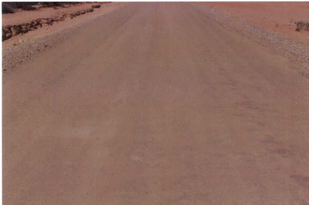
Photo 36. Undisturbed surface of Section 18 after 30 days
