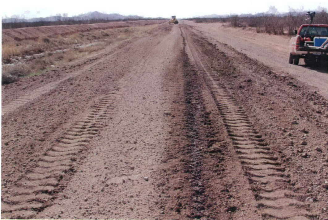
Photo 18. Dry center of test section and uneven product distribution after spreading of windrow on Section 5
