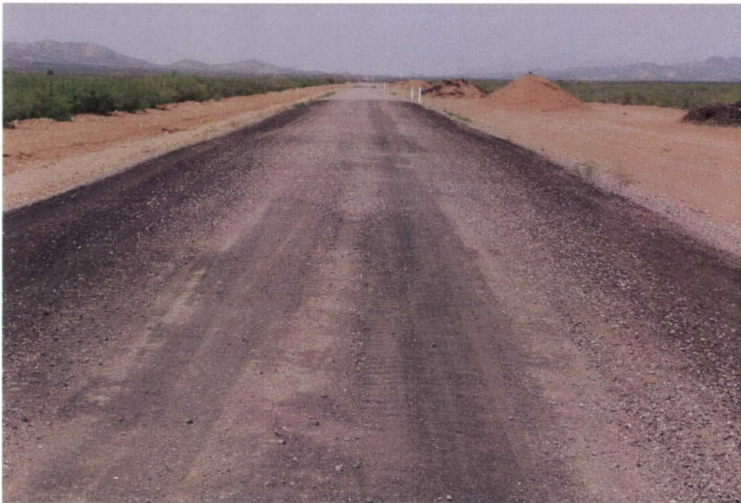
Photo 38. Disturbed surface of asphalt emulsion on Section 23 after 30 days
