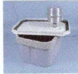
Above: Photos of vault housing the sensor, digitizer and RF modem.
