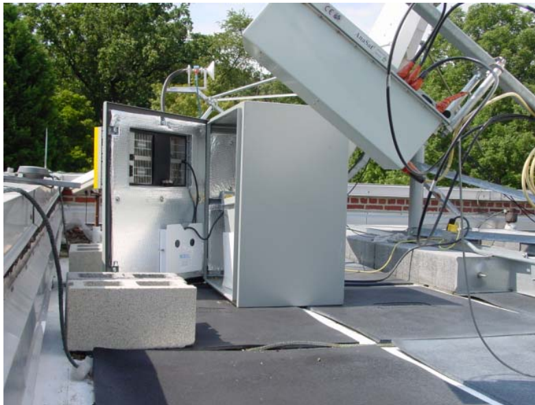
Figure 8. Thermoelectric all-weather chamber for TWSTT electronics.
