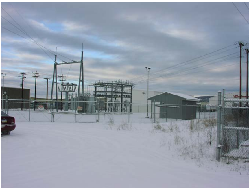
Figure 10. Standard 20 MVA GVEA substation.
