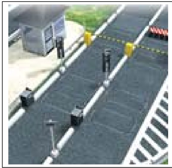
Figure 1. Unmanned Smart Gate with vehicle barrier.
