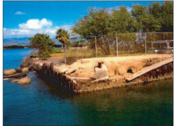
Photo 10. Deteriorated steel sheetpile bulkhead.
