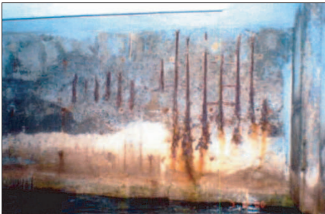
Photo 11. Spall along the face of the concrete curtain wall fronting the existing steel sheetpile wall.
