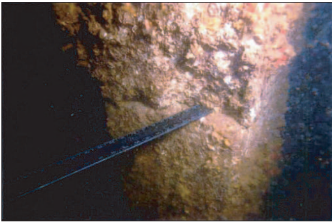
Photo 7. Fracture in pile.
