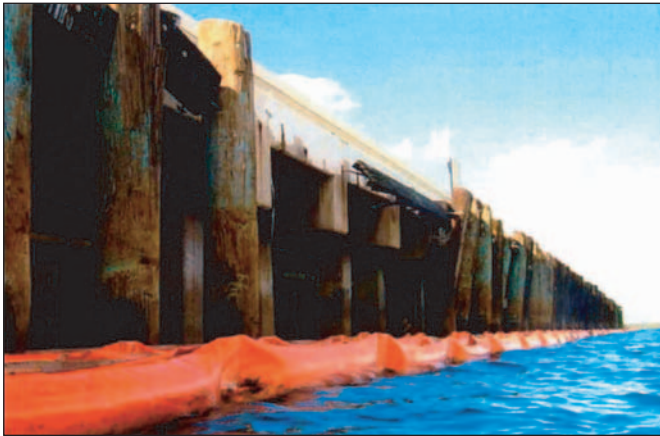
Photo 9. Deteriorated fender system.
