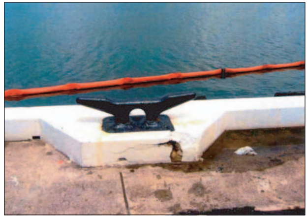
Photo 8. Spalling and delamination in the curb at 42-in cleat.
