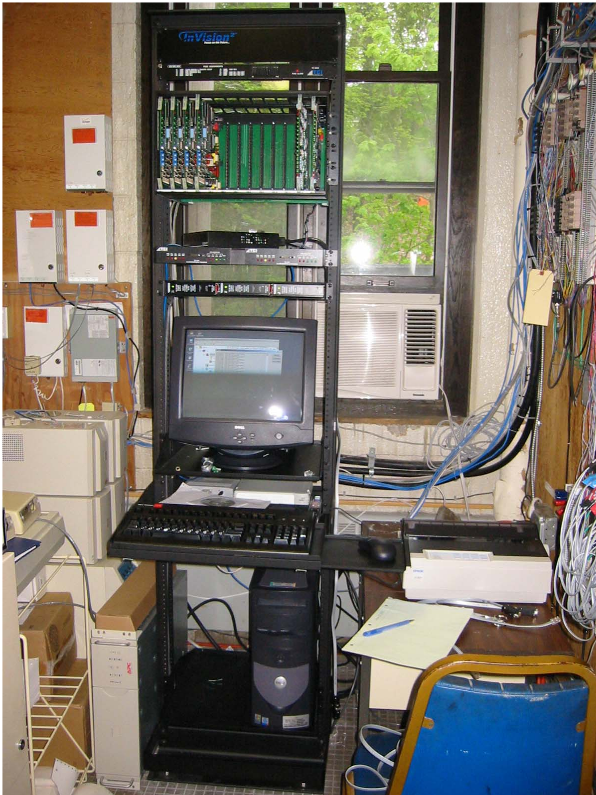
Figure C-11. Server Rack in Telephone Room.
