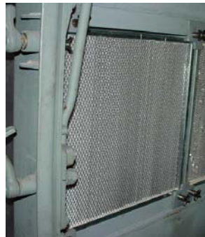
Figure 3. 2000 CFM LP HEPA Filter Installed
