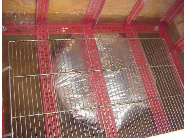
Figure 23. Figure 22: Close-up of immersed filter set.
