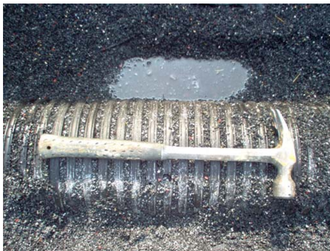
Figure 50. Puddle of Water at Lane 53.
