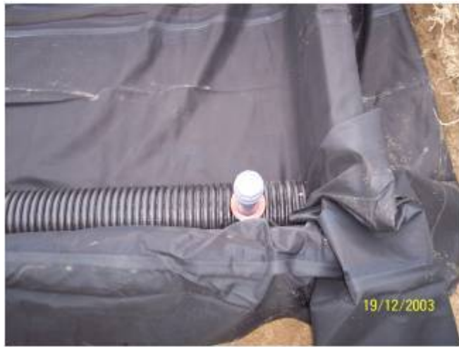
Figure 19. View Port of Water Collection Reservoir.
