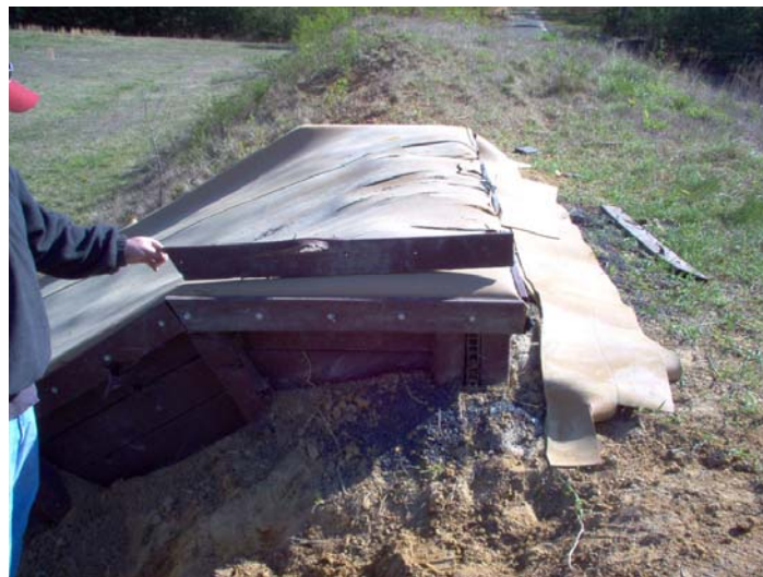
Figure 41. Damaged Frame/Plank Above-Replacement in Place Below.
