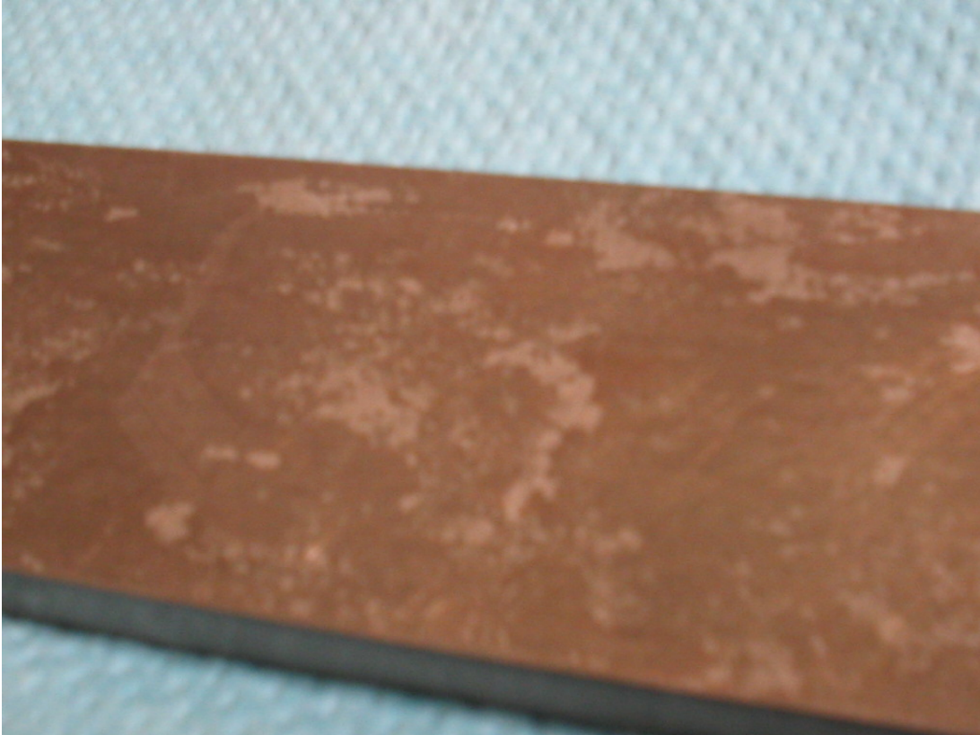
Figure 218. Zoom in on front of yellow/blue notched beam after corrosion and cleaning
