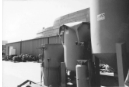
Figure 6: Abrasive Recycling Equipment Used in Demonstration
