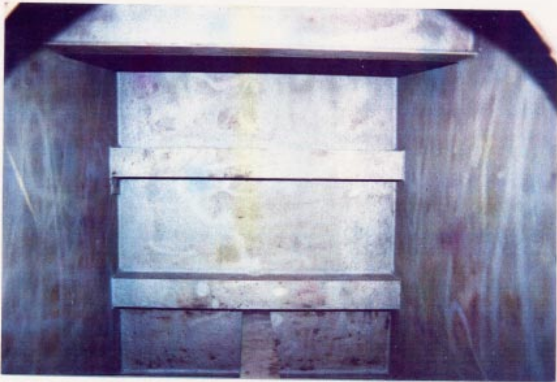
PHOTOGRAPH 4- NEAR WHITE CLEANED SURFACE SHOWING FLASH RUST
