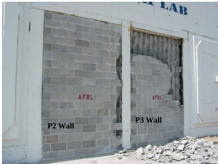
Figure 5.20 – Exterior of CMU Wall after Explosion
