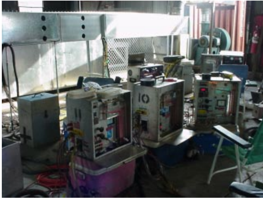
Figure 3: Sample Duct and Equipment
