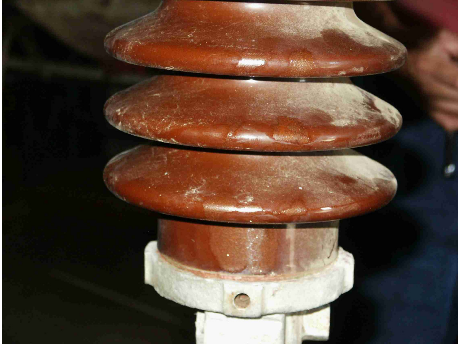
Figure 9. Insulator showing damage to glaze.
