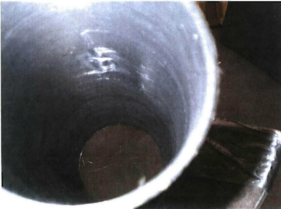
FIGURE H-11. Middle Hanger Failure (With Release), Inside View.
