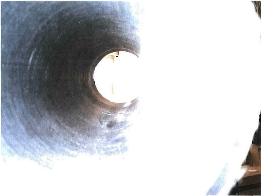
FIGURE J-11. Middle Hanger Failure (With Release), Inside View.
