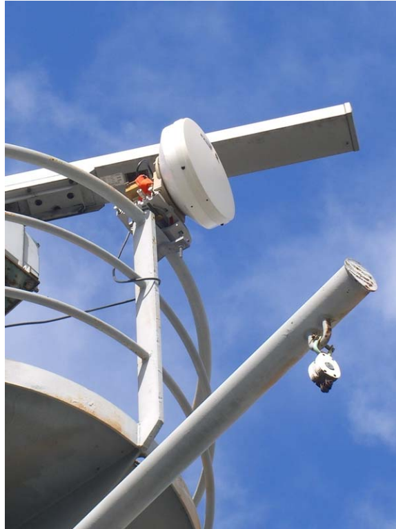
Figure 11. 802.16 Directional Antenna on the Navigation Radar Mast of GEM STATE (GEM STATE – USCG Island 802.16 PtP Link)
