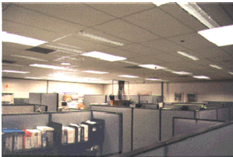
Figure 25. Office lighting tubes.
