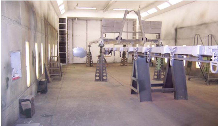
Figure 41. Large drive-in paint booth.
