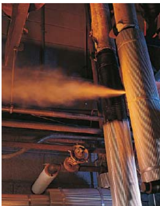
Figure 18. Large steam leak.
