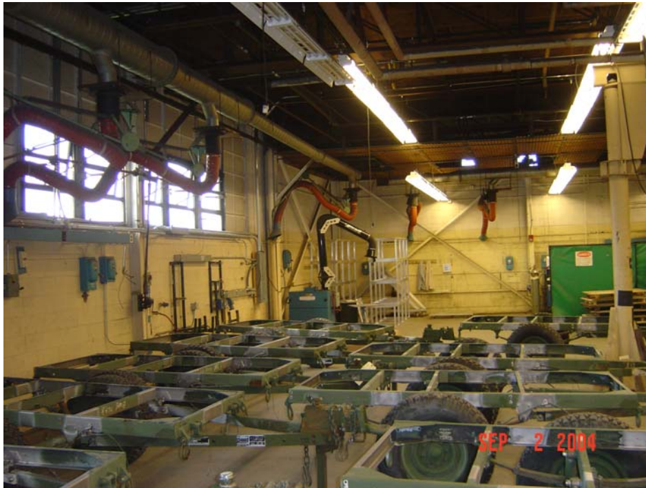
Figure 62. Storage area served by welding exhaust system.
