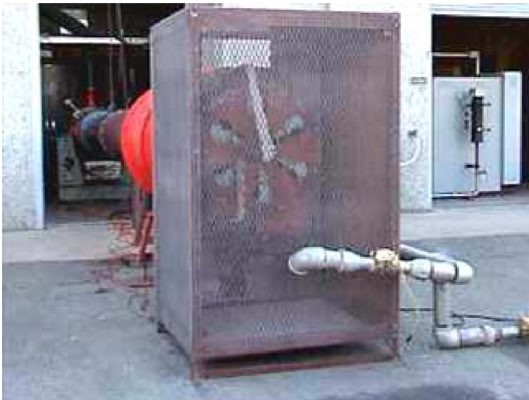
Figure 7. Steam pipe with intake plenum orientation (From Ref. 8)
