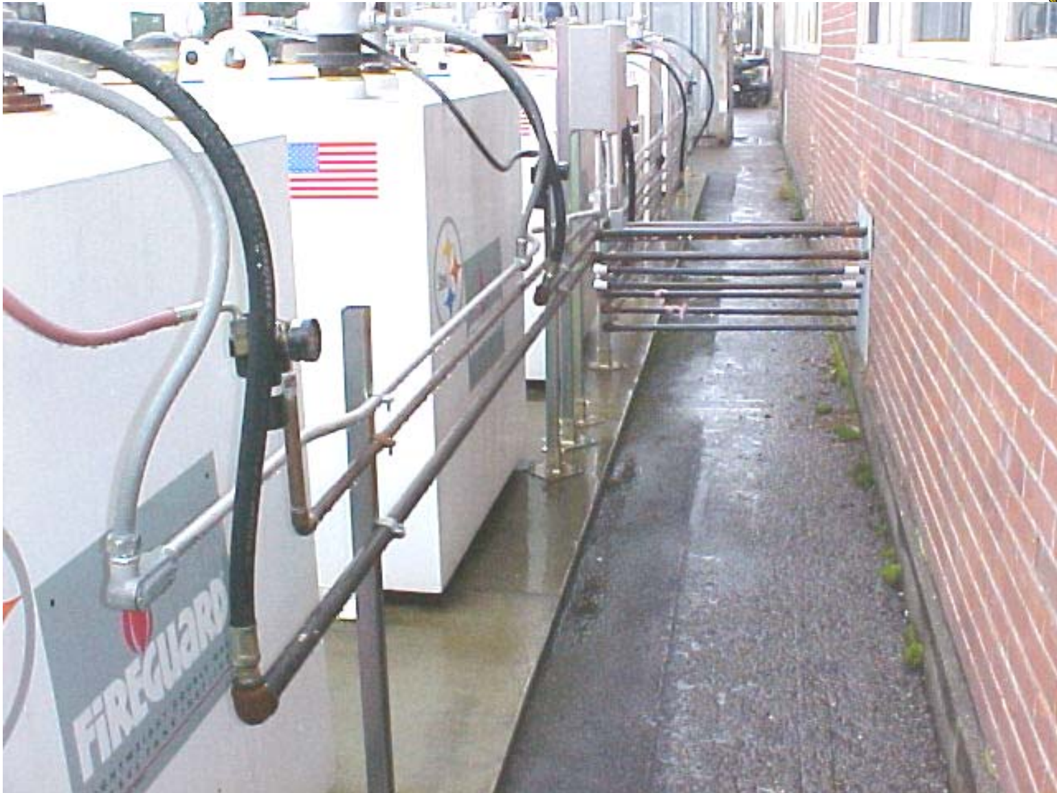
PIPING FROM STORAGE INTO BLDG 9580
